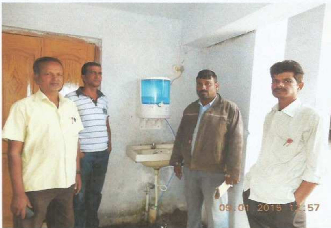
Aquaguard fitted in the school of Sri Aurobindo Integral Education & Research Centre, Matrubhumi, Dera, Talcher by Global Coal & Mining Pvt. Ltd.
